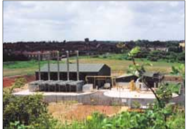
Figure 9. Shirebrook CMM gas project (courtesy of Clarke Energy Ltd)
