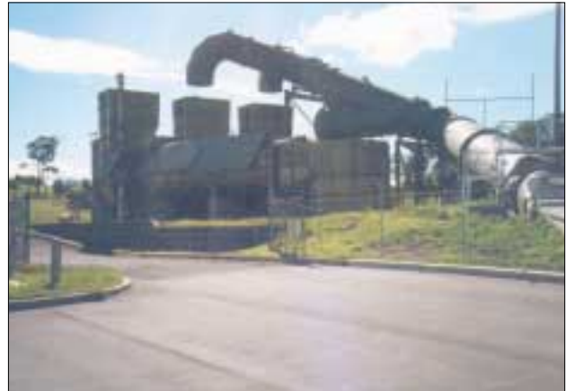
Figure 4. Ducting methane in ventilation air for combustion in gas engines at BHP's Appin Colliery, Australia (courtesy of Wardell Armstrong)
