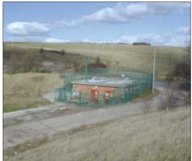
Figure 10. Silverdale gas compression station at Stoke, UK (courtesy of Octagon Energy Ltd)
